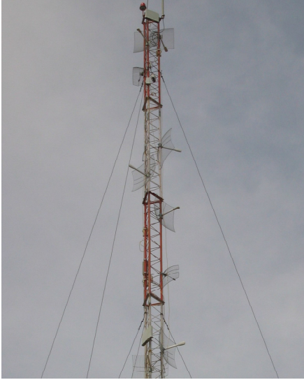
Figure 2: Picture of a radio tower in the Akshaya [2] deployment featuring multiple antennas for point-to-multipoint connectivity. The antennas need to be aligned on the vertical axis and aimed carefully.
