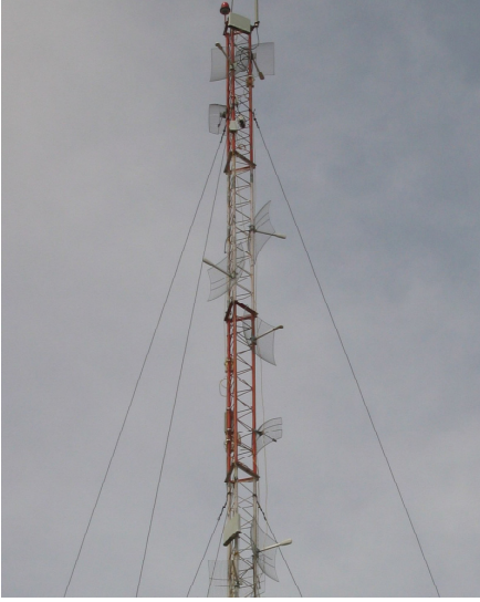
Figure 2: Picture of a radio tower in the Akshaya [2] deployment featuring multiple antennas for point-to-multipoint connectivity. The antennas need to be aligned on the vertical axis and aimed carefully.
